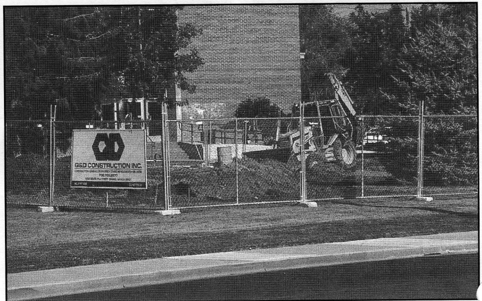
Construction begins almost immediately, as seen in this photo, taken in September 1999.
